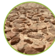
Deep exposure. Exposure depth approx. 4 mm
