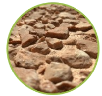
Deep exposure. Exposure depth approx. 6 mm
